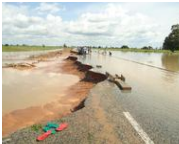
Figure 2.1. Unmaintained highway in the North–East region (Numan-Biu- Maiduguri road)
